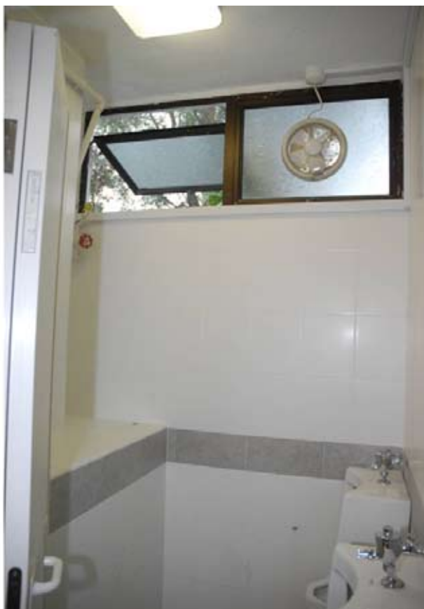
Urinal Cubicle with Ventilation Window opened
